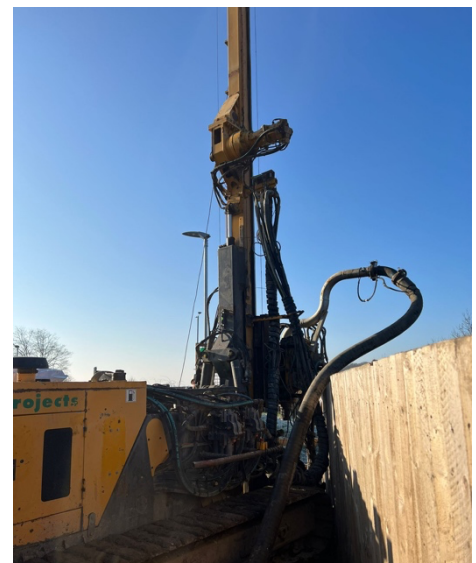
Figure 2: The Klemm 709 Piling rig, ideal for piling in areas where space is tight.
